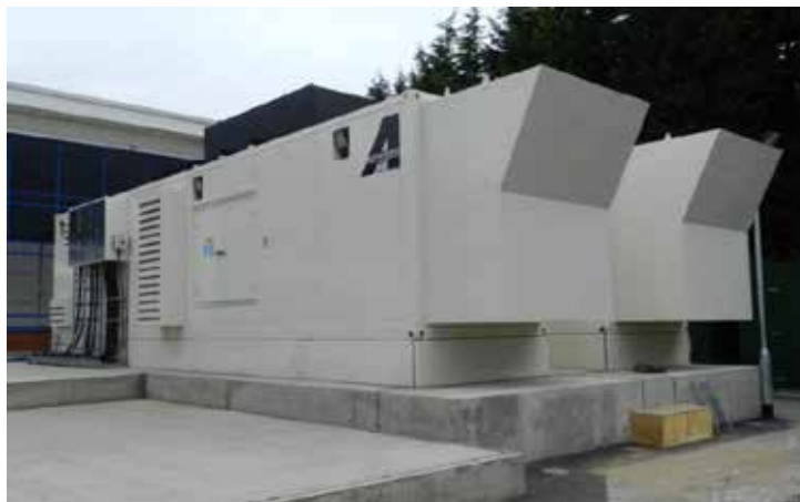
The co-operative bank 3 x 500 kVA n+1 www.co-operativebank.co.uk
